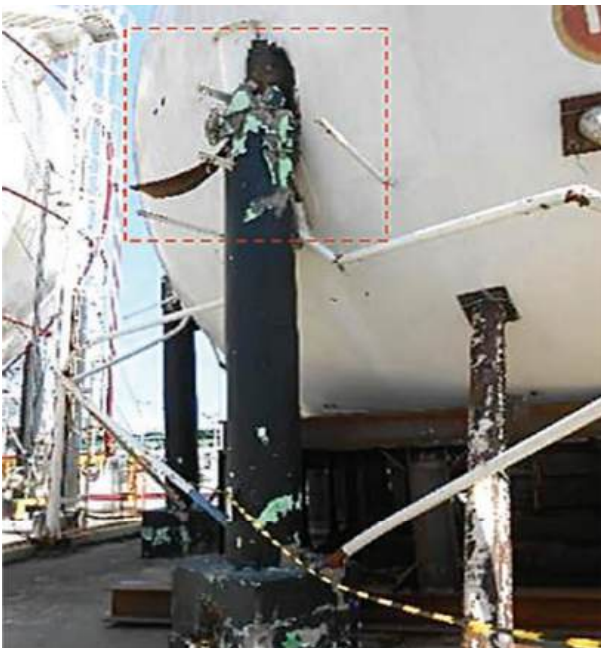
Figure 1 Damage to one of the supporting structures of tank T-1B (Dyah et al., 2016)
