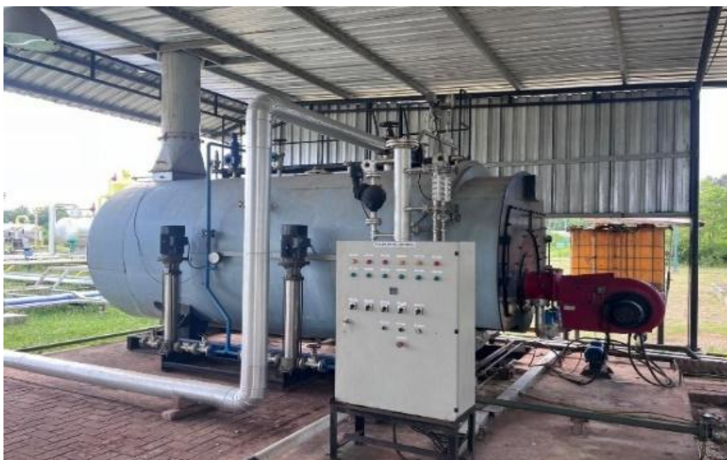
Figure 4. Dual fuel water boiler.
