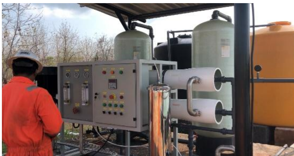
Figure 3. Reverse osmosis water treatment as boiler inlet.
