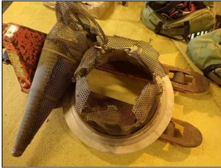
Figure 1. Strainer conditions during operation show catastrophic failure, leading to debris pass-through and potential downstream component damage.
