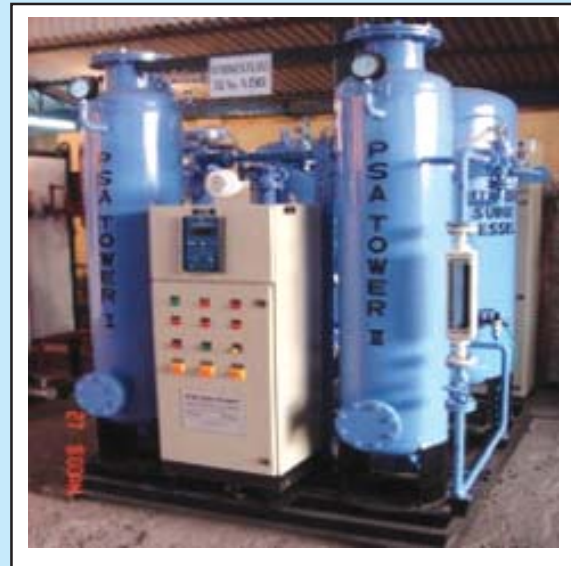
Gambar 3 PSA Generator model skid mounted [2]
